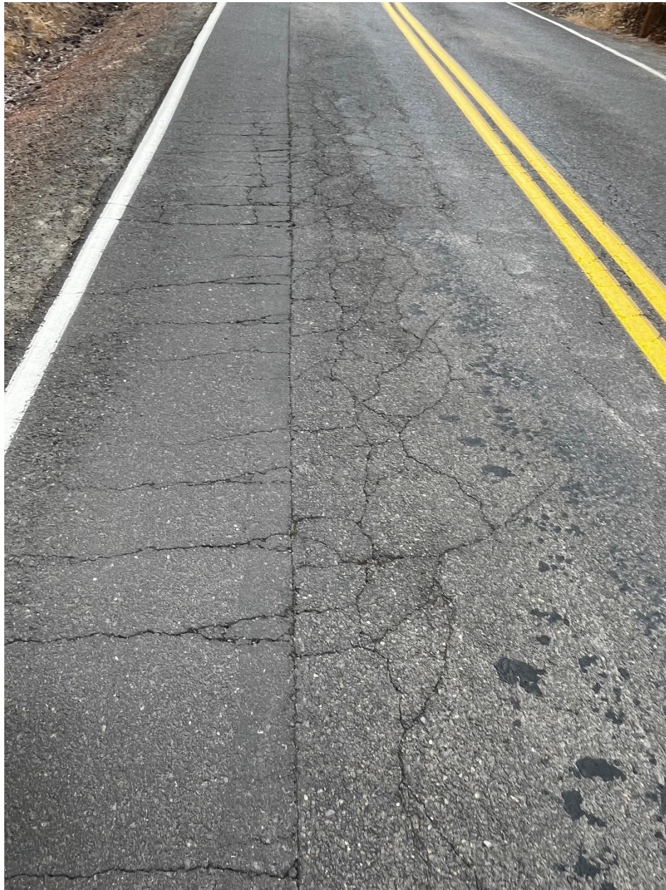
Additional documentation of degradation of Powers Ave.
